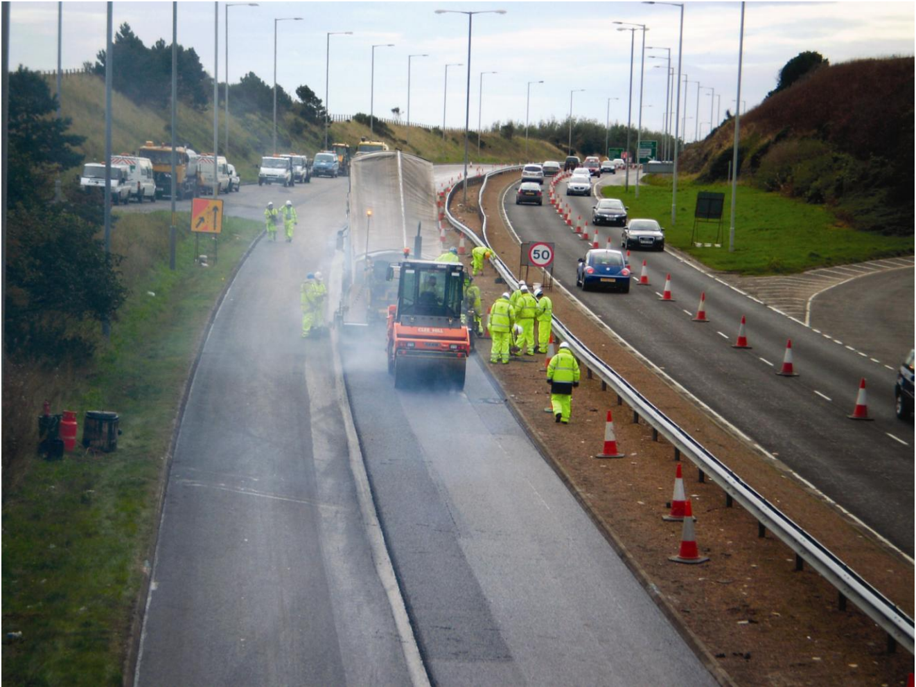
Leiths' reconstruction of the A90 in Aberdeenshire achieved excellent skidding results with high performance binders in lieu of high friction surfacing
